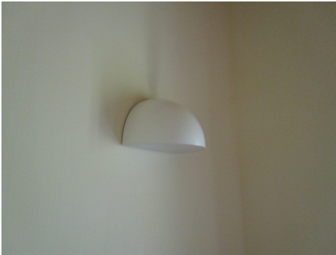
殆どの照明器具 Most light fixtures
